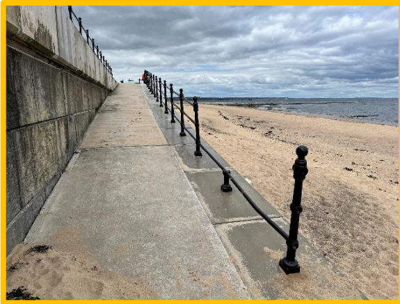
Damaged handrail on access ramp at Vane Street (/C0303C01)
