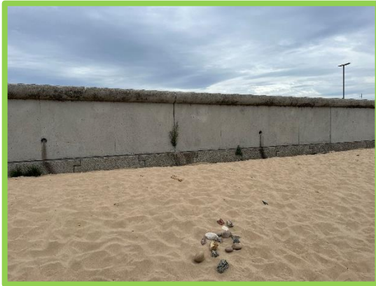
Vegetation growing in joints – should be removed (/C0501C04)
