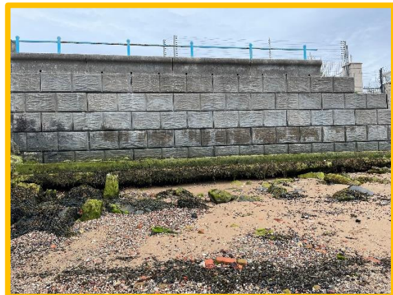
Low beach levels exposing undercutting of concrete toe to the west. (/C0401C27)
