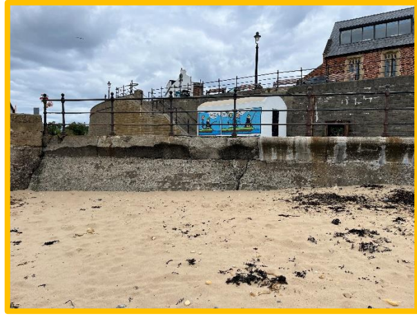
Spalling damage to recurve wall, significant crack suggesting settlement. Old Pier to left of image (/C0401C05)
