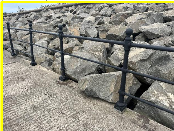
Displaced rock damaging handrail (/C0401C33)
