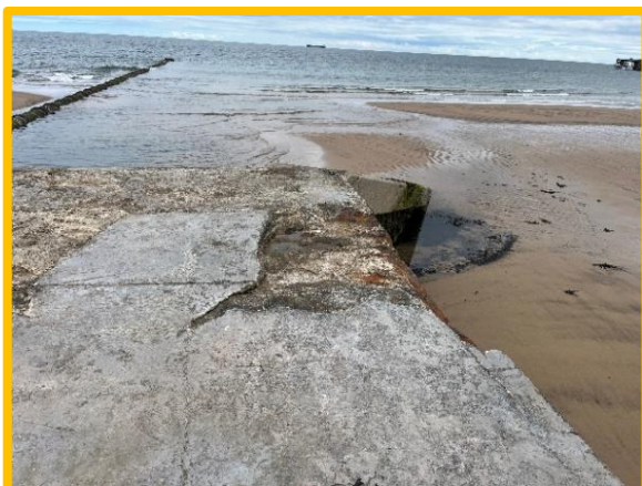
Cracking / spalling to piled outfall structure deck (/C0302C01)
