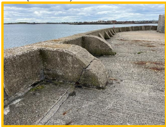
Cracking in parapet wall and deck (/C0401C34)
