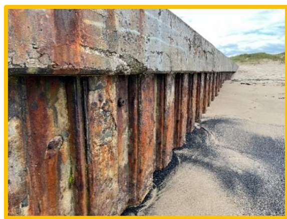
Heavily corroded piled outfall structure (/C0302C01)
