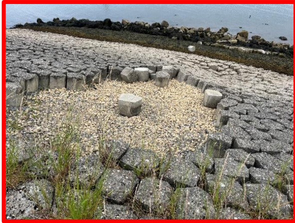
Unravelling of concrete blockwork revetment (/C0401C26)
