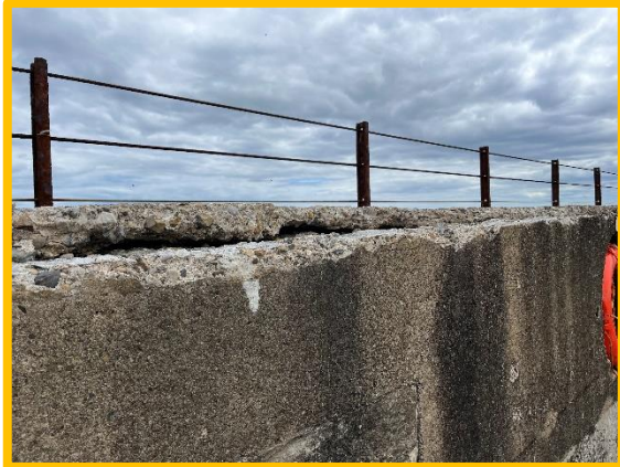
Spalling of concrete (/C0401C01)
