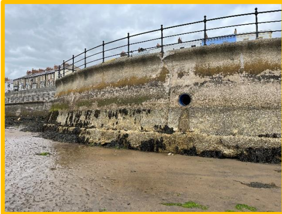
Damaged cope around handrailing fixing (/C0401C04)
