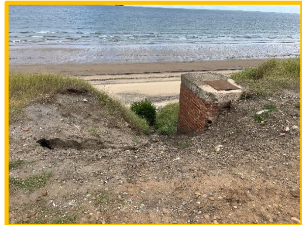
Manhole chamber at risk due to ongoing erosion (/C0302C01)
