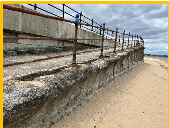
Damaged cope to Thorpe Street access ramp (/C0303C01)
