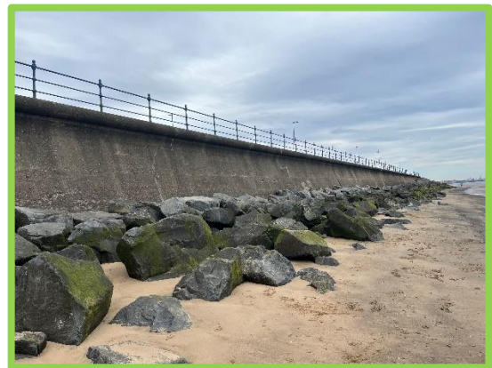
View looking north. High beach levels concealing toe of revetment structure. (/C0501C05)
