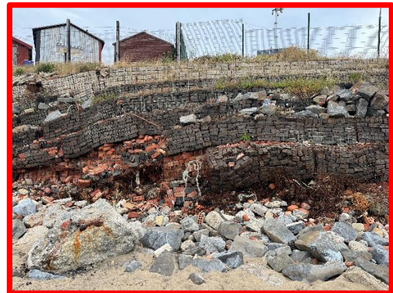
Stacked gabion wall in very poor condition especially to the south (/C0401C17)
