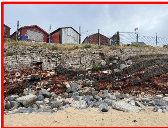
Stacked gabion wall in very poor condition especially to the south (/C0401C17)
