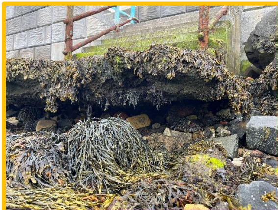
Undercutting of access steps (/C0401C27)
