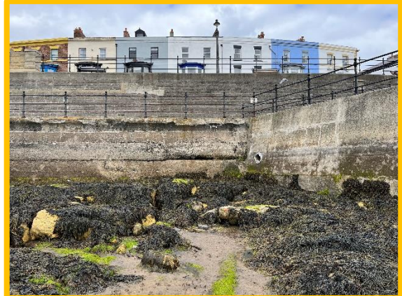
Broken Flap Valve (/C0401C04)
