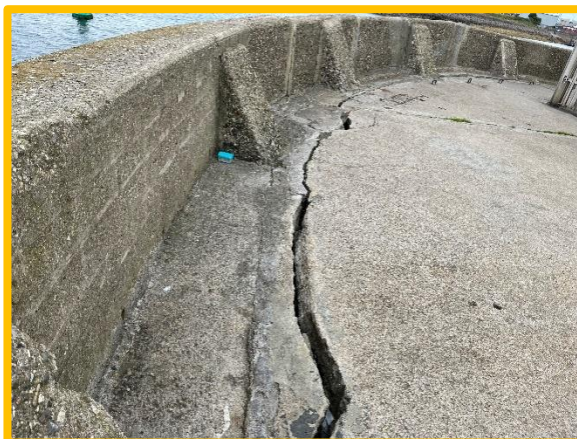
Cracking in parapet wall and deck (/C0401C34)
