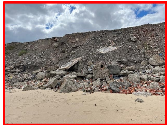
Burst brick gabions spread along foreshore to the north (/0302C02)
