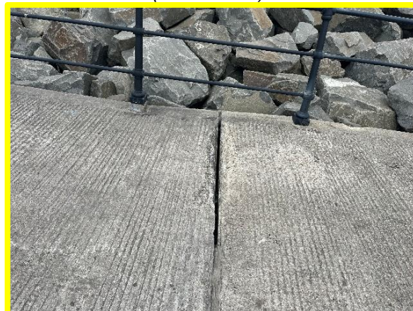
Loss of flexible joint sealant in northern access ramp, potential trip hazard (/C0401C33)
