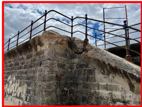
Local damage to coping/handrails at Thorpe Street access steps (/C0303C01)
