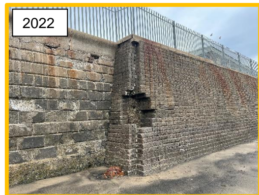
Progressive loss of blocks at interface between two walls. (/C0401C19)
