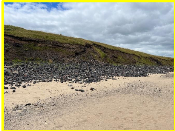
Historic slipping in coastal slope (/C0302C03)
