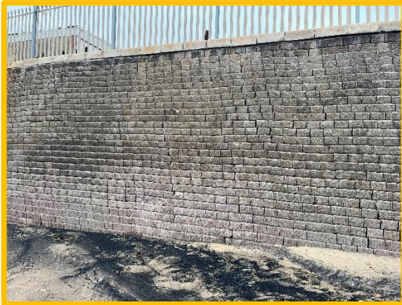
Inconsistent profile, missing copes, open joints (/C0401C19)
