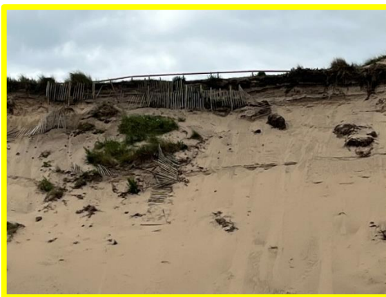
High, steep, unvegetated dune with eroding crest adjacent to Crimdon Beck (/C0301C01)
