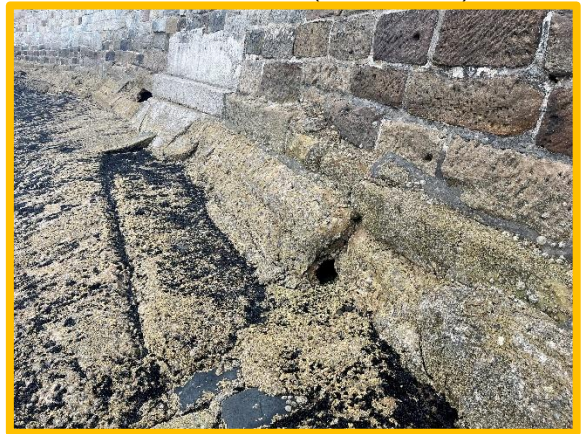
Voids observed in toe of north face of North Pier(/C0401C22)
