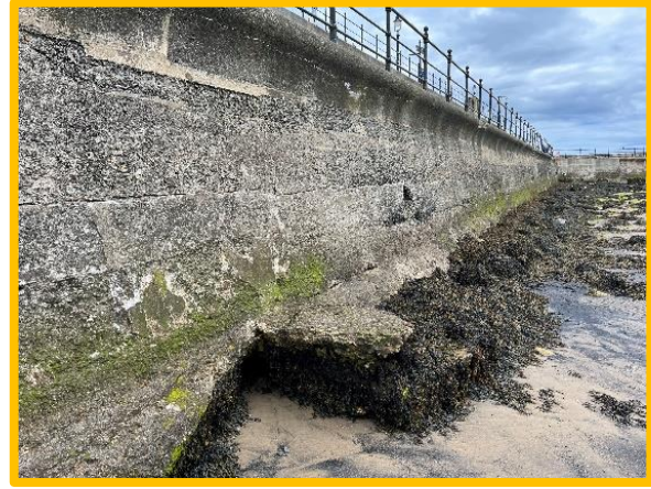
Voiding at toe of wall (/C0401C05)
