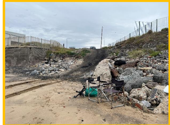
Erosion outflanking seawall at Informal access ramp (/C0401C18)
