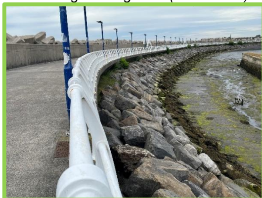
Inner face of South Pier. Vegetation can be seen on crest. (/C0401C32)
