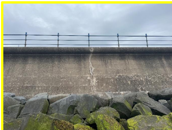
Vertical cracking through cope and wall (/C0501C05)
