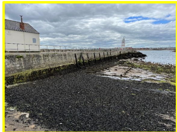
Inner face of North Pier – uneven profile suggesting potential settlement of masonry blocks (/C0401C06)
