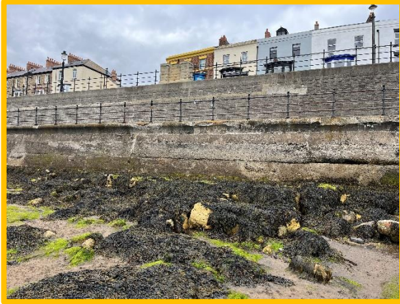
Damaged recurve cope (/C0401C05)
