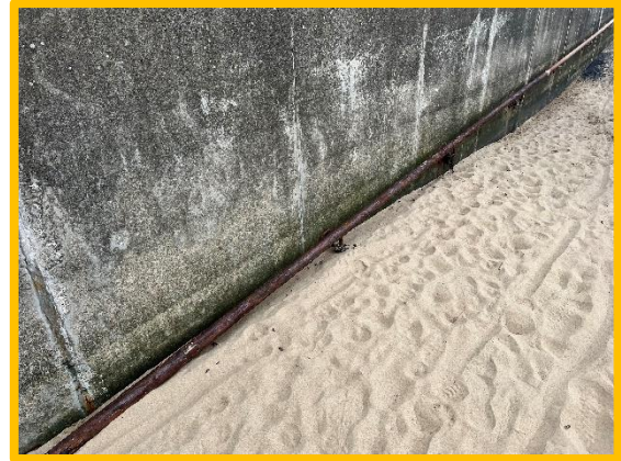
Heavily corroded handrail on lower section of ramp (/C0401C33)
