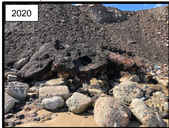
Erosion of made ground slope in 2020 (/C0302C02)
