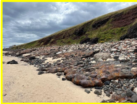
Deteriorating slag-poured apron (/C0302C03)
