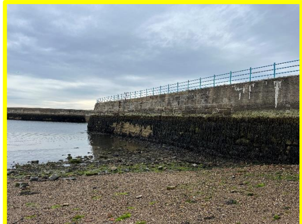
Inner face of Middle Pier heavily vegetated (/C0401C28)
