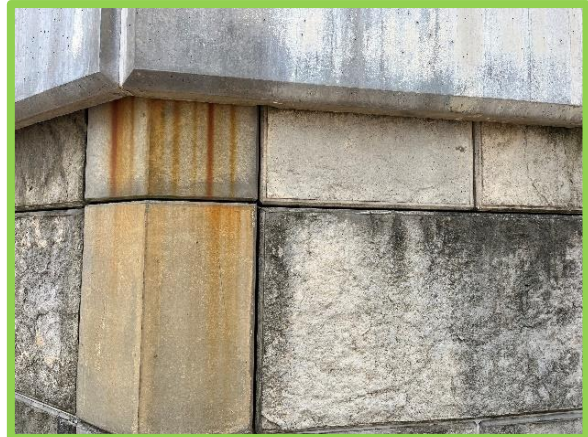
Sealant being washed out between precast units (/C0303C01)
