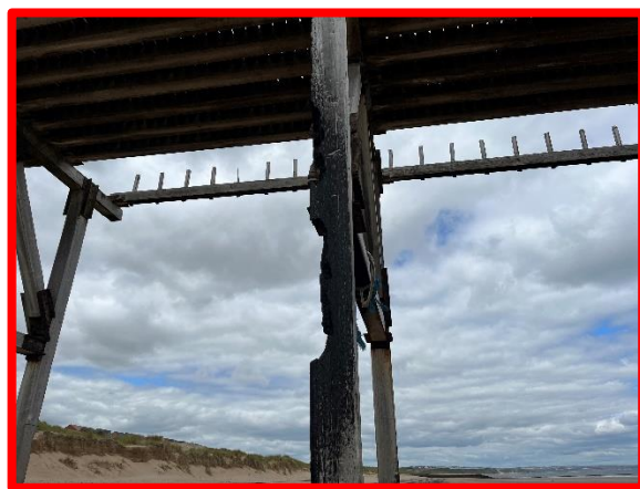
Loss of section to timber support columns of historic pier structure, likely due to fire damage (/C0302C01)
