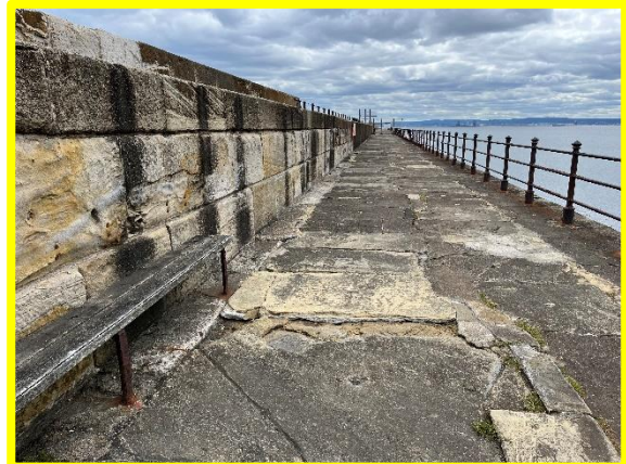
Cracking to the deck slab (/C0401C01)
